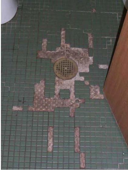
Kit Anderson House - Broken and missing bathroom tiles
