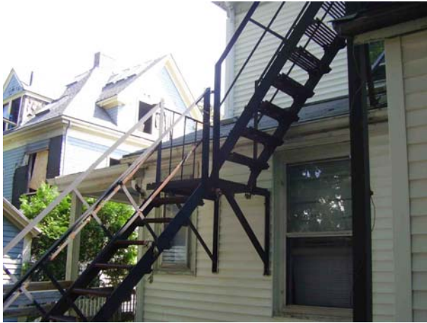
Old and rusty fire escape
