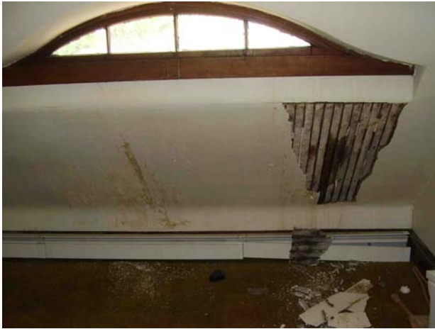
17 Monmouth St - Water damaged and crumbling walls
